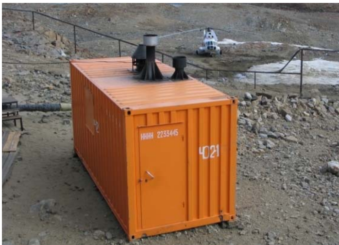
Figure 1. Incinerator module at Novolazarevskaya station
