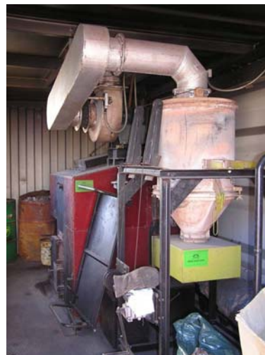
Figure 2. Incinerator IN-50 at Progress station
